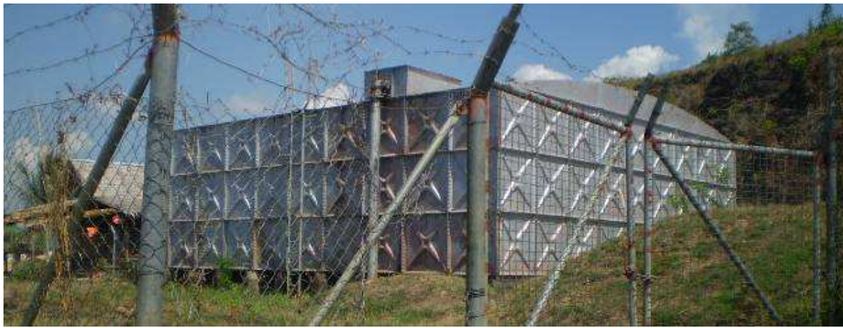
Plate B-2: A water tank at the back of Honiara
